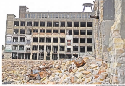
The former Mirro manufacturing plant in downtown Manitowoc sits in a state of rubble and disrepair in this 2015 photo. The rest of the structure will be demolished beginning April 11.
