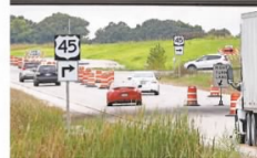
VEHICLES ENTER AND EXIT STATE HIGHWAY 151 AT THE HIGHWAY 45 INTERCHANGE. THE INTERCHANGE FOR U.S. 45 AND U.S. 151 OPENS FULLY FRIDAY EVENING.
